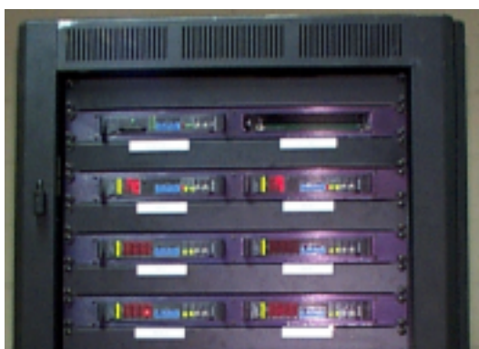
Centralized Show Control System: 128 digitals, 32 analogs, 208 lighting
