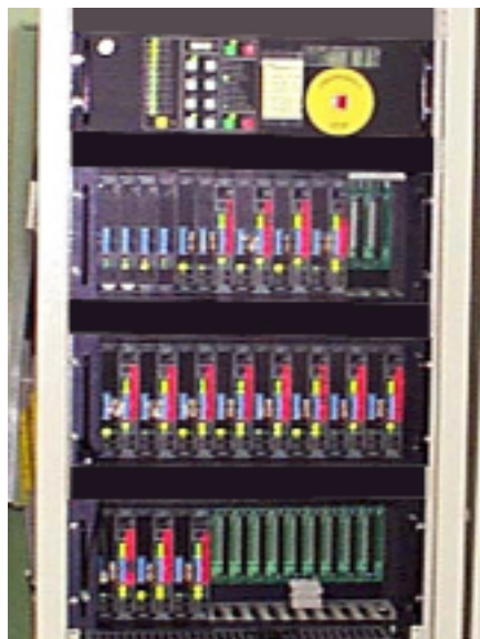
Centralized Control System w/ Kp-300 Operator Panel: 132 Digitals, 415 analogs, 240 lighting
